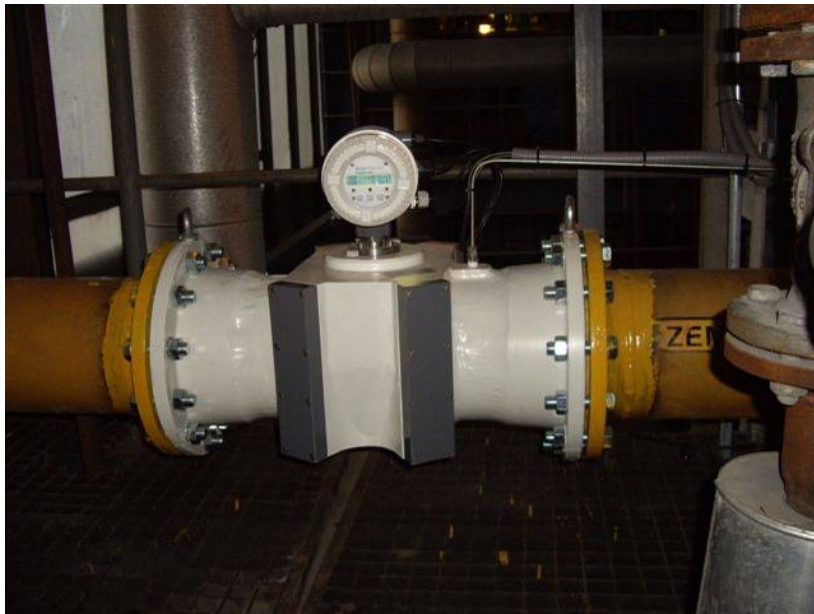
Fig. 11: Meter installation for 13 psig fuel gas measurement
