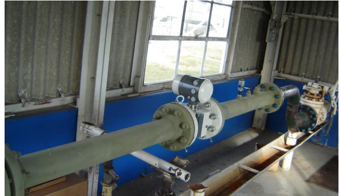
b) meter and downstream piping
