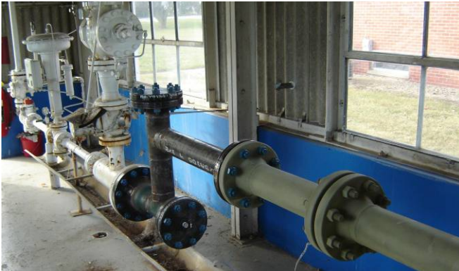
a) Regulator and upstream piping
