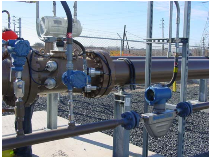
A 1/2" Coriolis and 12" ultrasonic in a fuel gas metering installation.
