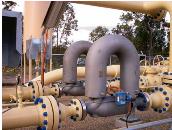
100mm (4") Coriolis meters installed in 250mm (10") lines
