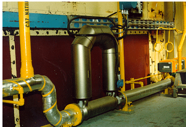
Combustion control application to boilers
