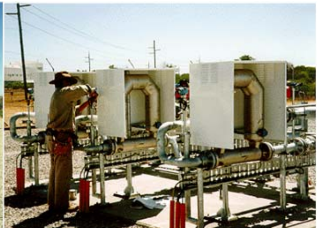
"After" installation since 1996, with operating and one "hot spare" meter
