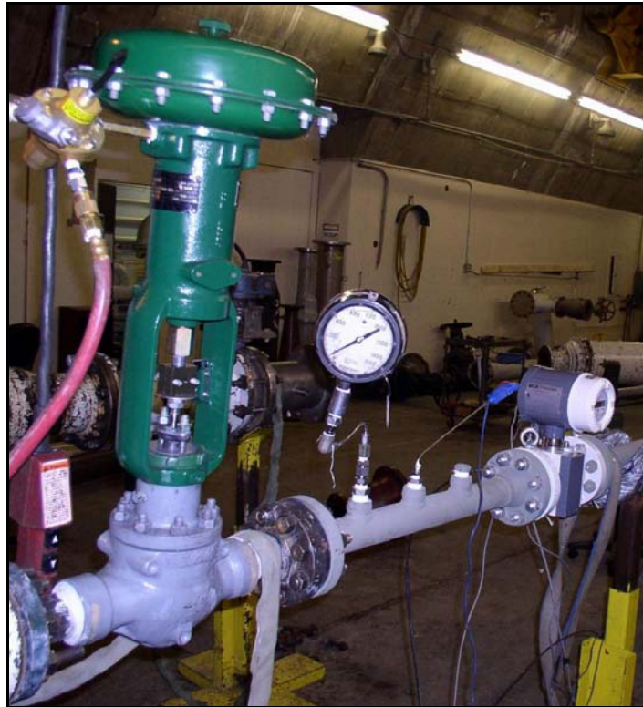
Figure 14 – Control Valve Piping
