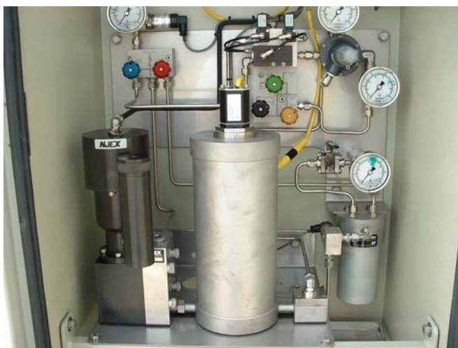
Figure 1; Injection Pump and Meter
