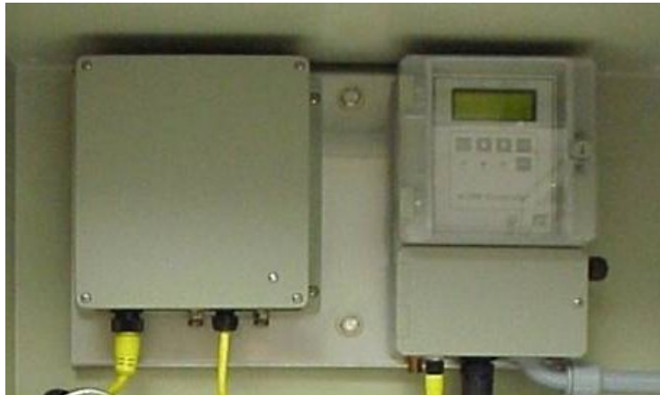
Figure 2; Injection Rate Controller
