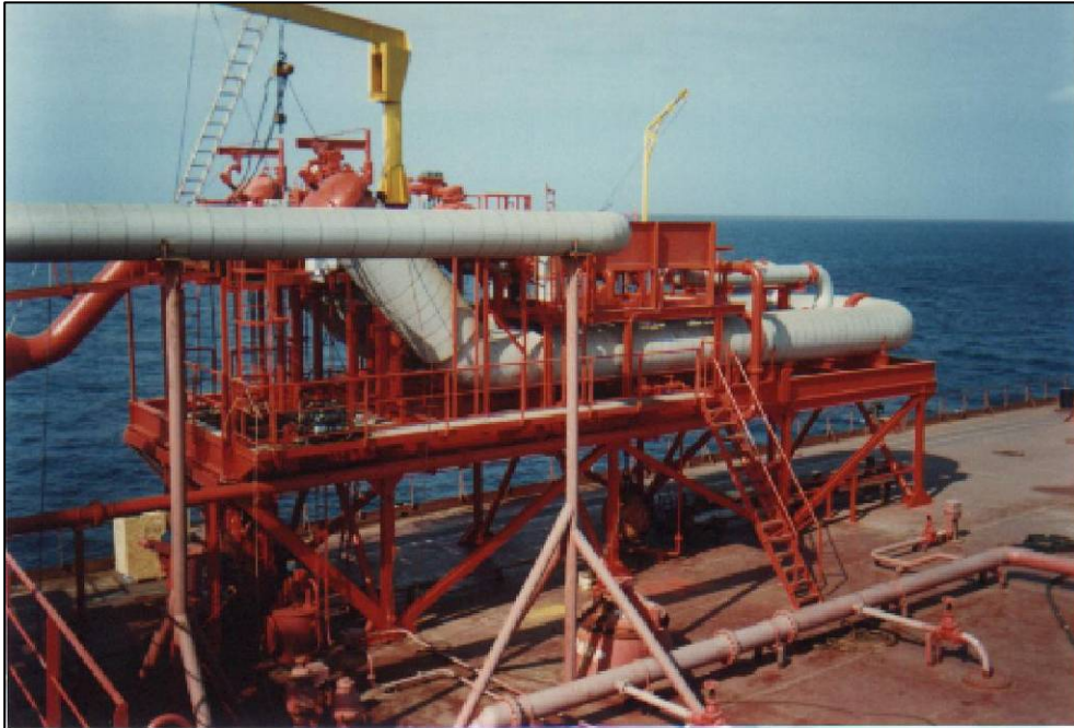
Fig 3 42" Prover on an FPSO
