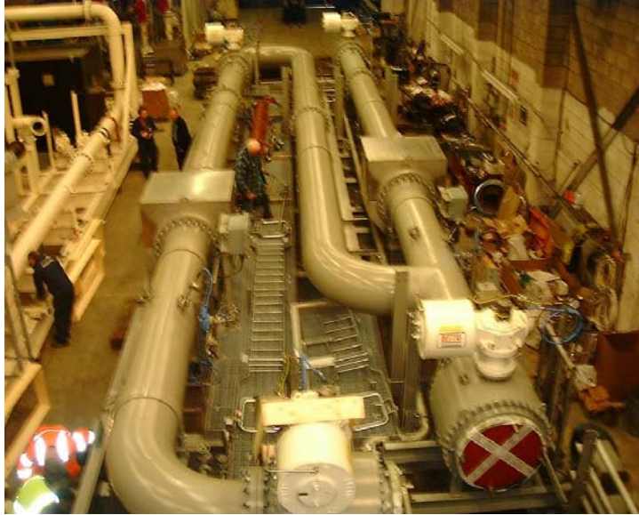
Fig 7 Offline Master Meter Installation
