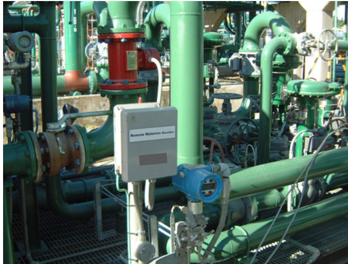
Figure 3.0 Flow Computer for a CTM application also used for BS&W Application
