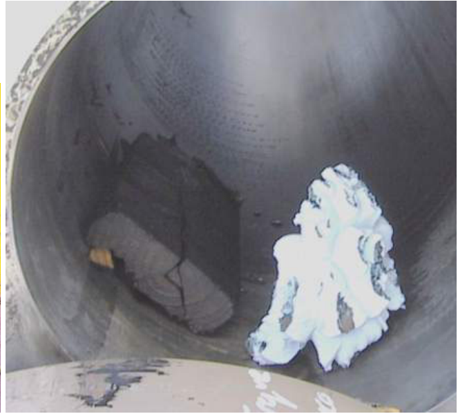
Figure 25 – 12-inch Flow Conditioner Blockage
