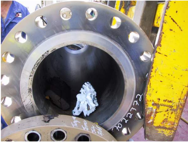
Figure 24 – 12-inch Flow Conditioner Blockage
