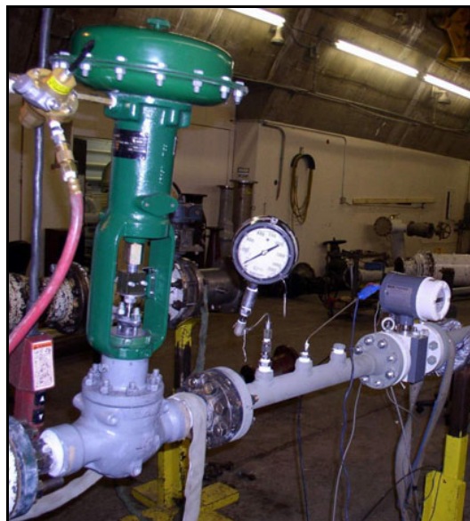
Figure 8 – Control Valve near 2-inch USM
